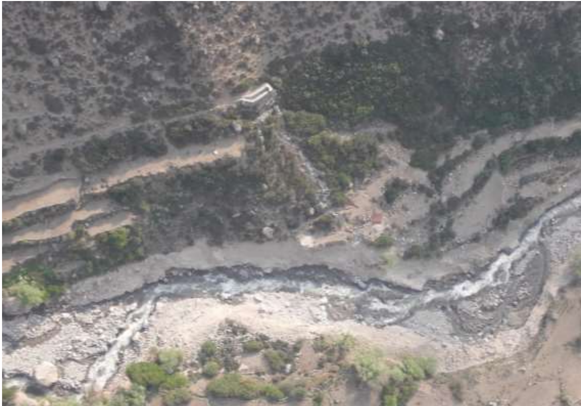
Figure 9. Photo from the UAV showing the 15KW HP Powerhouse washout area including the collection of penstock pipes impacted by the flood. (Source: Sudan Bikash Maharjan).
