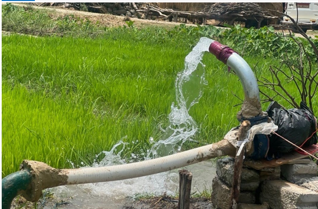
FIGURE 1 ELECTRIC MOTOR WATER PUMP THAT REDUCES FARMER'S WORKLOAD WHILE INCREASING ACCESS TO IRRIGATION
