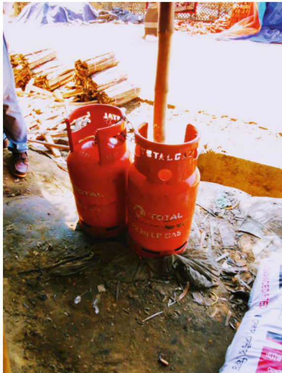
Fig. 12.3 LPG distribution centres inside the camps. Photograph credit A. K. Enamul Haque
