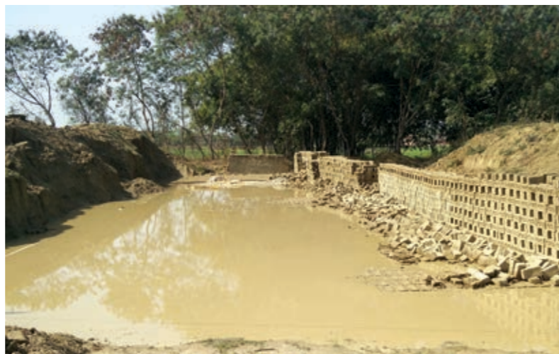
BRICKS DAMAGED BY THE PREVIOUS NIGHT'S RAIN
