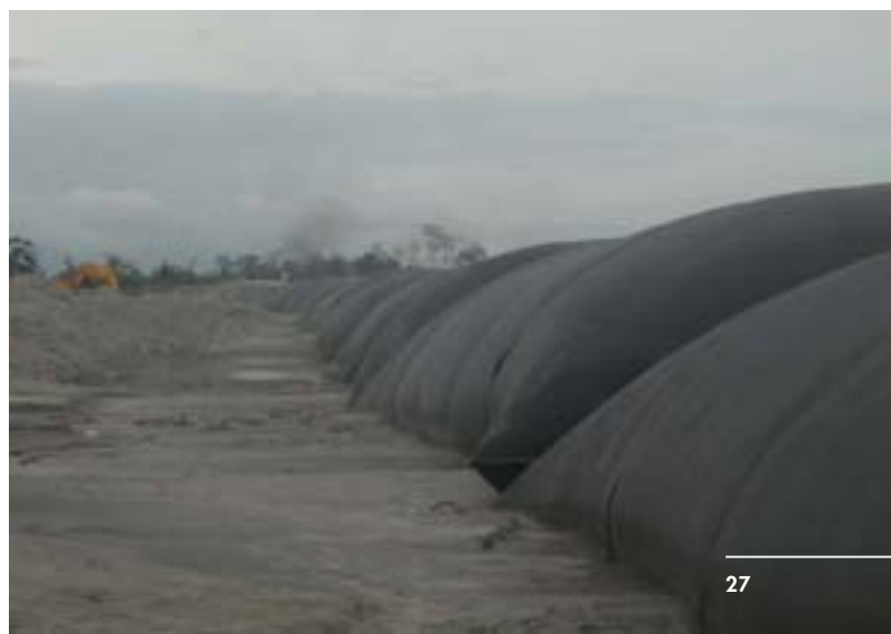
Figure 14: The last hope: ongoing construction of the new embankment in Matmora where geo-tube technology is being used for the first time in India.
