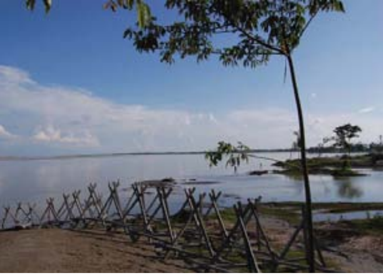
Figure 22: Away from us! Holding back the river with porcupine anti-erosion measures at the breached portion (eastern) of the Matmora embankment
