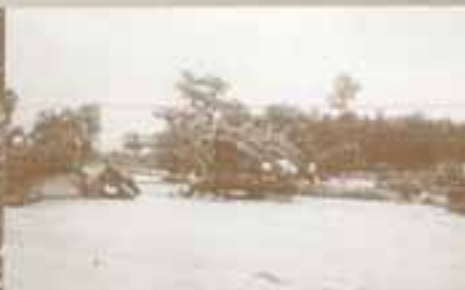
Bridge damaged by the Pampa Khola in Aug 2001 in Kathar VDC of Chitwan District
