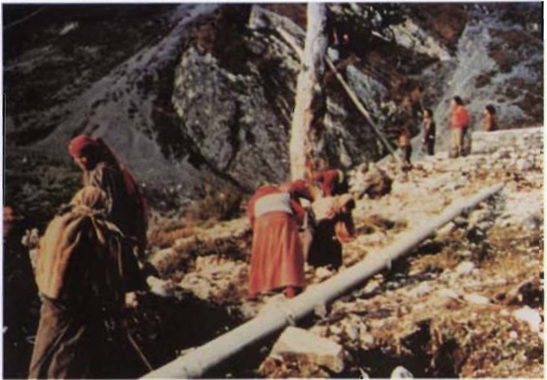
Village labour: the use of local labour and skills not only reduces costs but also ensures community commitment to the project.
