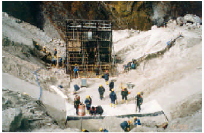
Figure 12.3: Gate structure with partially erected gates. In the foreground geomembrane and geotextile are being laid (photo credit: Shrestha 2000)
