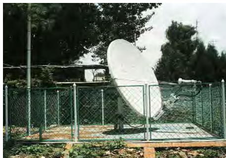
Mercure earth station
