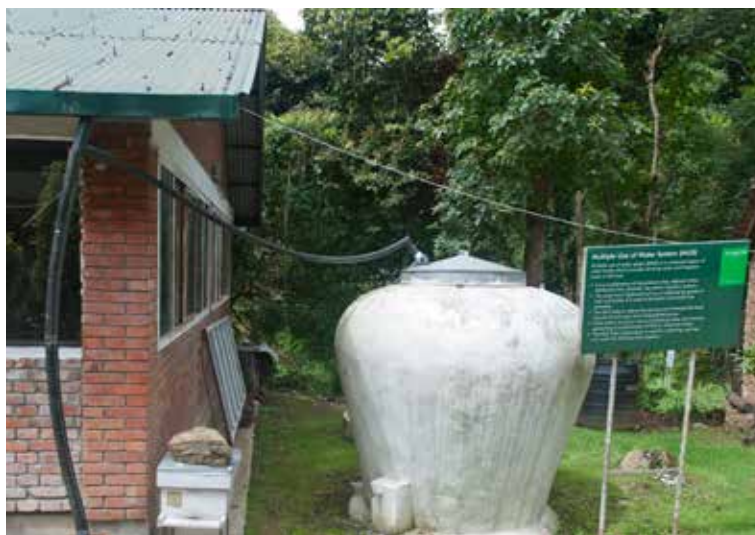
Roof top rain water harvesting (Ferro-cement jar)
