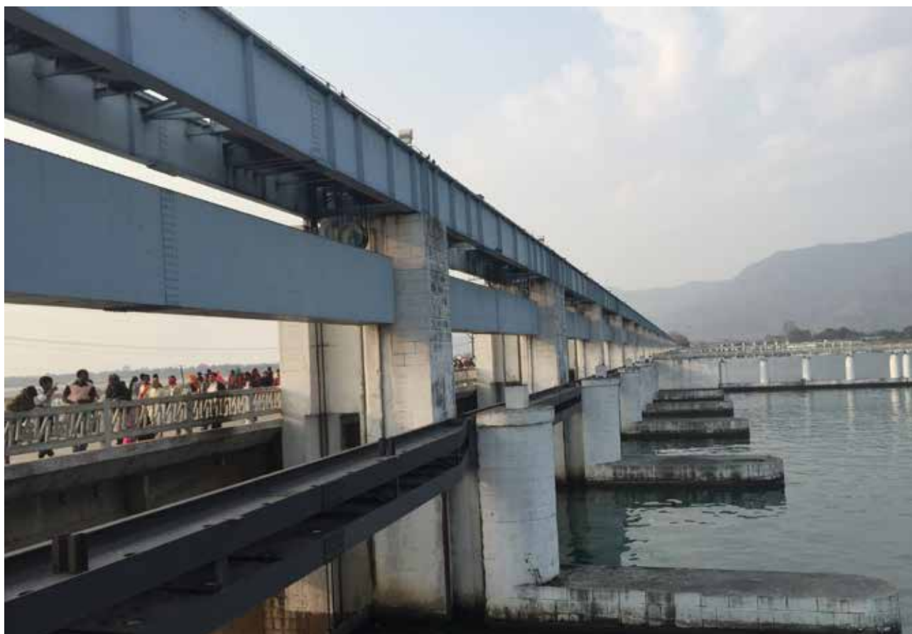
Road linking India and Nepal over the Gandak Barrage on the Nepal-India border
