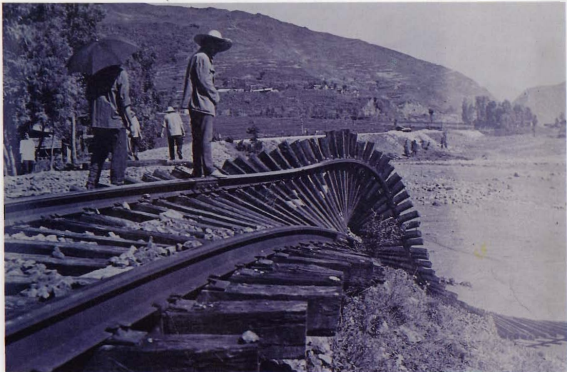
The embankment was undermined by debris flow and flooding following breaching of a debris flow dam formed on 30 June, 1981. Courtesy of Yang Wenke
