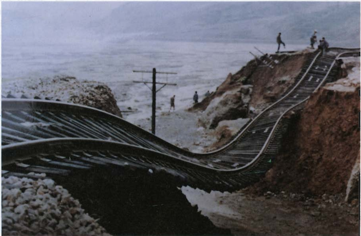
Plate 3: Debris Flow Undermining the Embankment of Dongchuan-Kunming Railway (1 July, 1985)
