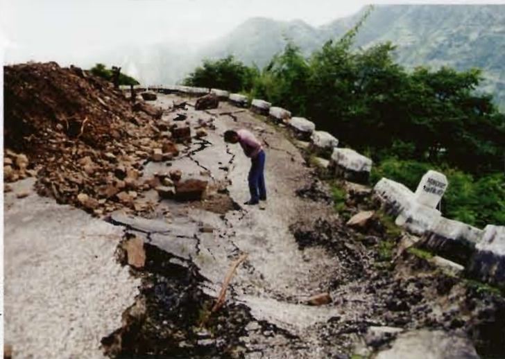
Damage to the Dharan Dhankuta road by 21 August 1988 earthquake, Nepal
