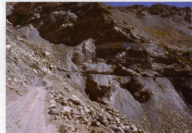
Himalayan roads constantly face the danger of landslides. Here, a 100-meter section of road in Lahaul district slipped away, causing vehicular traffic to detour over 500 kilometers.
