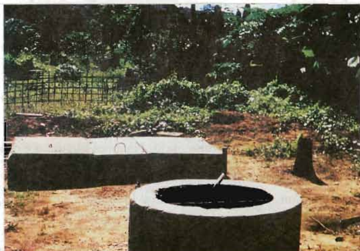
Dome-type biogas plant installed in the Panchkhal Valley, Kabhrepalanchok, Nepal
