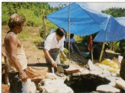
Figure 99: Mr. Xu Zhaokun Advising the Nepal Team on Construction of the Water Tank
